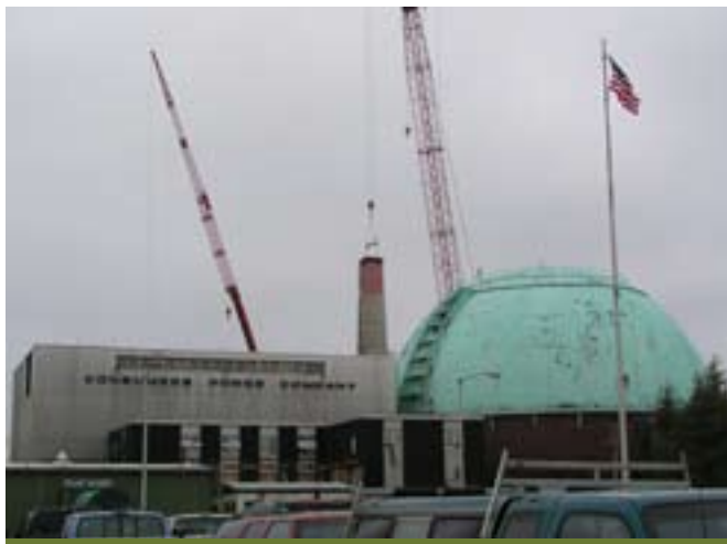
Big Rock Point Power Plant
