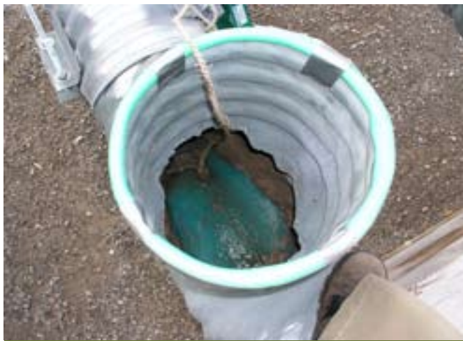
Floc Log Entry Port with 706 Floc Log Visible
