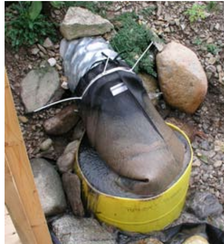
System Exit Point - Note 'black' [clarified] water
