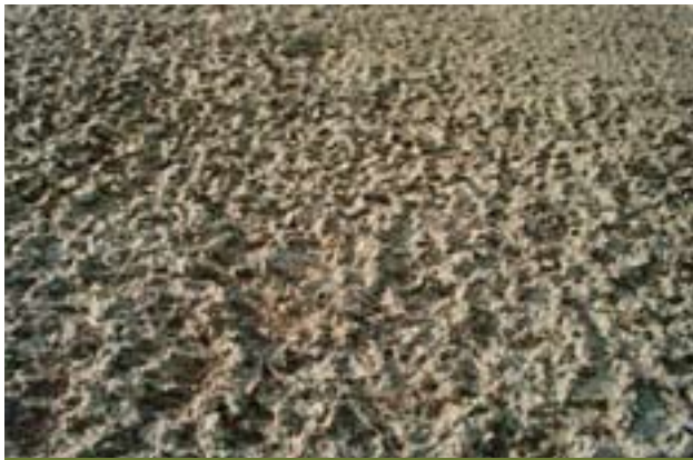
Mulch condition on slope after 1" rainfall
