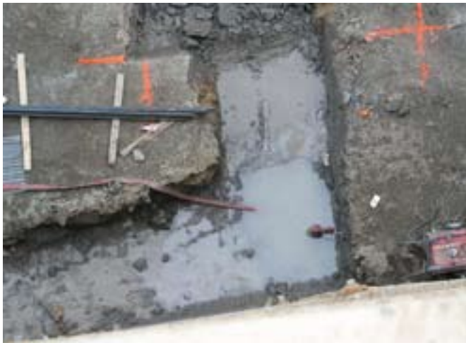
Excavation dewatering; red hose sends pump effluent to Floc Log clarification system
