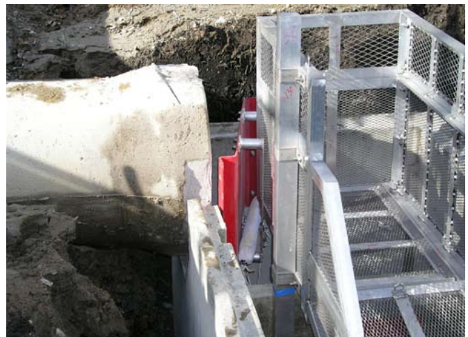
Outlet pipe orientation requires slanted skimmer placement
