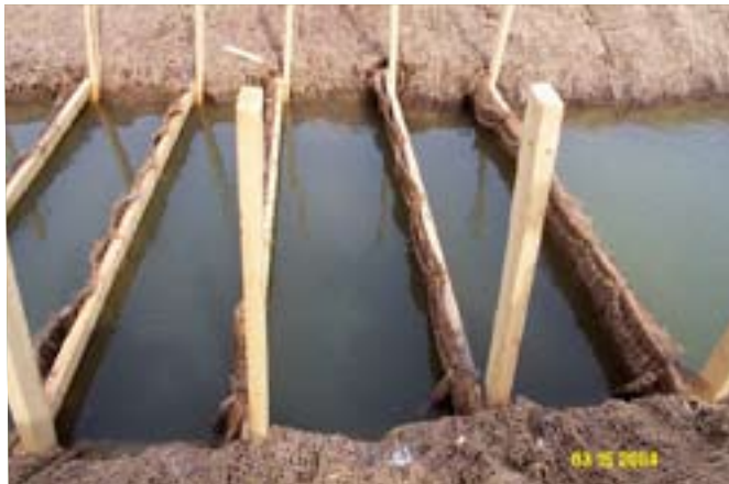
Baffle grid flow from right to left. Note: water clarity change
