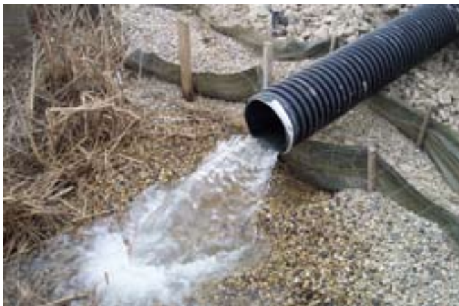
Discharge from Floc Log clarification system to adjacent wetlands
