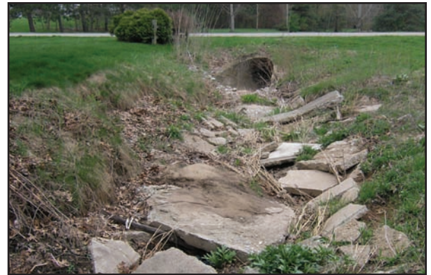
Before the re-design, the existing drainage channel was lined with broken concrete slabs, and erosion was occurring in the channel.
