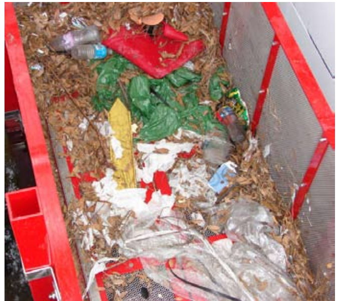
Vegetation & litter trapped in NSBB screen system
