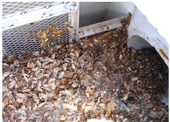
Basket system in need of maintenance
