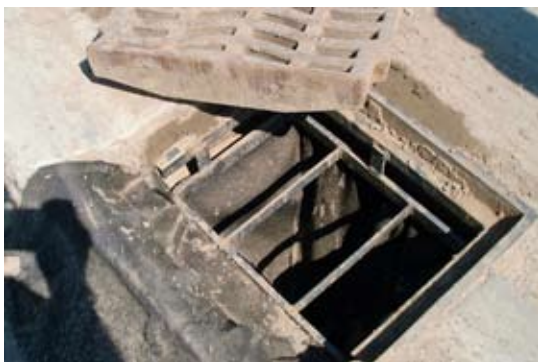
Installed Catch-All: Note overflow opening
