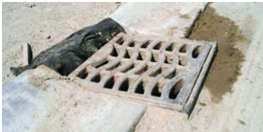
Installed Catch-All: Note little vertical grate displacement
