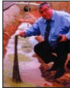
Environmental - Standing water can lead to poisonous green algae or other environmental hazards in road drainage.
