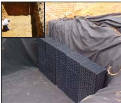
Minimum excavation was required to prepare the area for the RainTank system.
