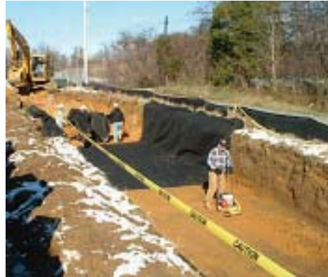
Use pins, rocks, or sandbags to prevent geotextile from sliding or blowing down into the excavation.
