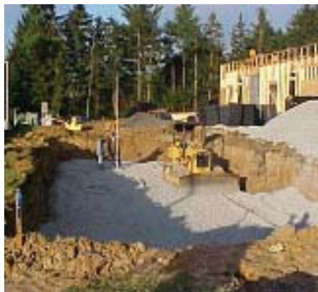
Establish a smooth and level working platform. Base depth is not critical but creating an even platform will make tank installation easier.
