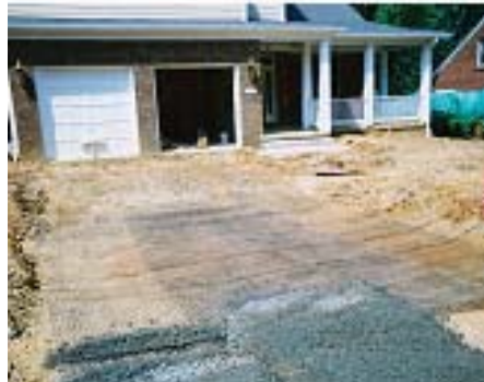
Extending the geogrid at least 3' beyond the excavation footprint will help prevent differential settlement.
