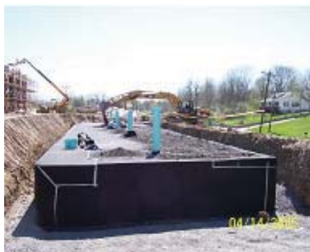
When folding geotextile around corners, make clean folds and secure with duct tape.
