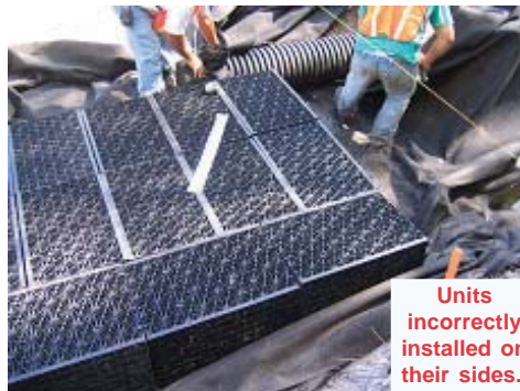
While the perpendicular row has been installed correctly, these units have been placed on their SIDES. This is evident from the lines formed by the edges of the top and bottom panels, which should NEVER be seen from the top.
