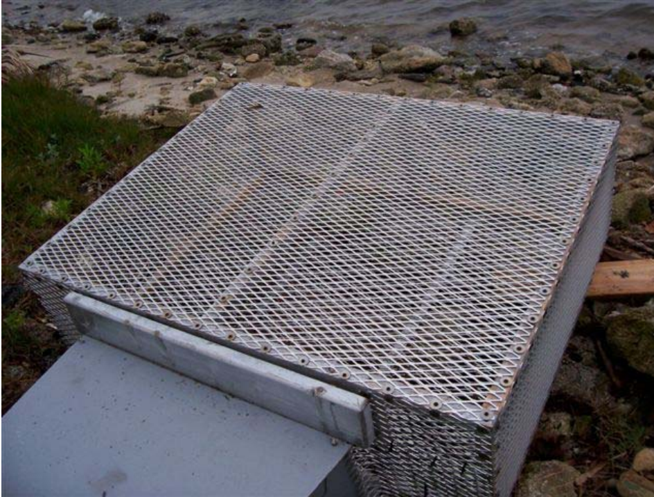
Figure 5. Effluent screen basket.
