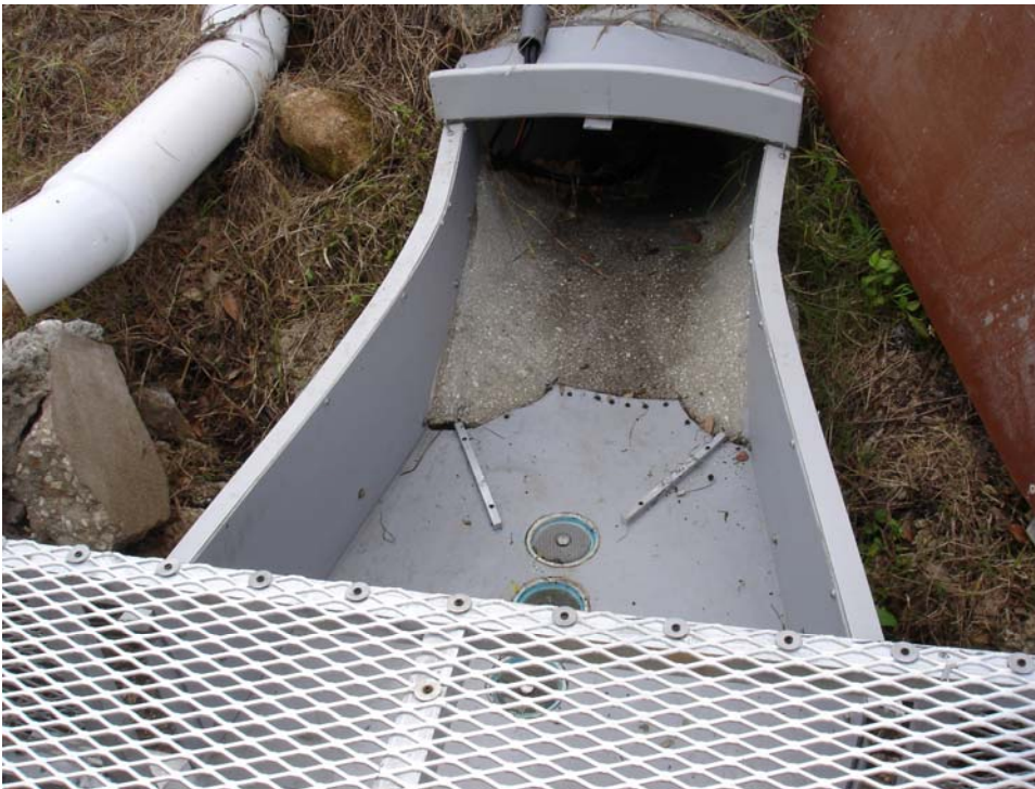
Figure 6. Flume connecting baffle box to effluent basket.
