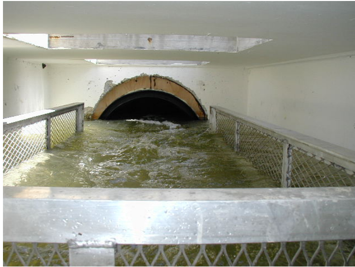
Inlet of Baffle Box with flow at 9000 GPM
