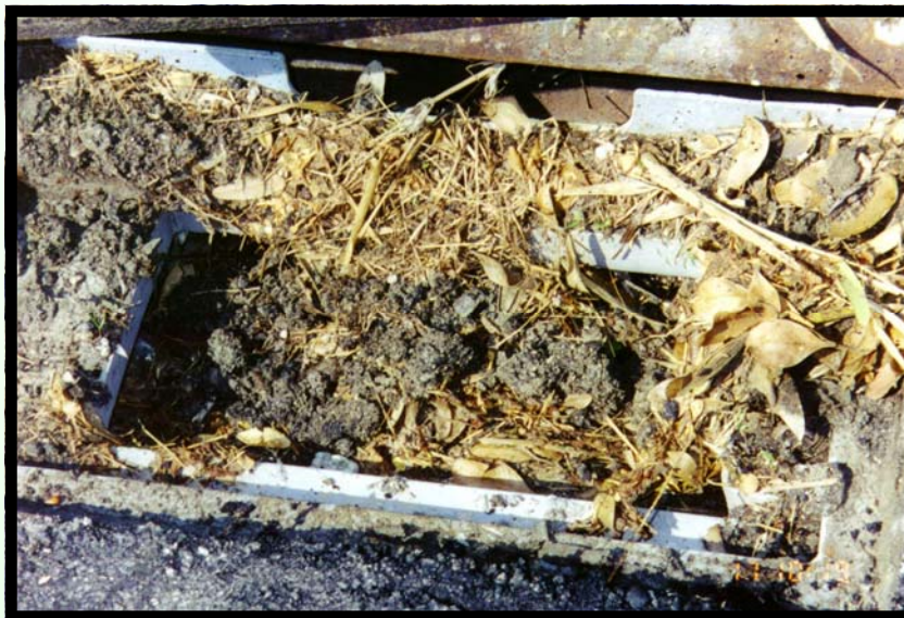
Above: Inlet immediately after the grate was removed. This Grate Inlet Skimmer Box measures only 11"
