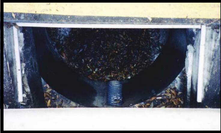
Left: The white battens attached around the catchbasin opening support the Grate Inlet Skimmer Box .
