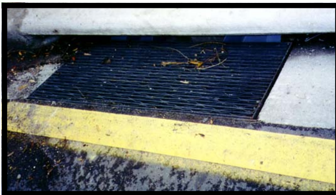
Above: View of grate in place over the Grate Inlet Skimmer Box , which is nearly invisible.
