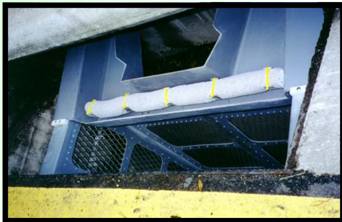
Above: View of the Grate Inlet Skimmer Box with flume, completely installed and ready for grate to be place back.
